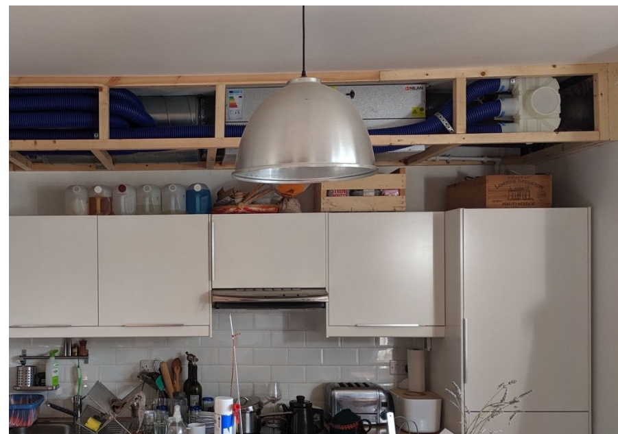
Installation of a whole house mechanical ventilation system with heat recovery in a flat as part of a retrofit. In this case installed in the ceiling above a kitchen.
