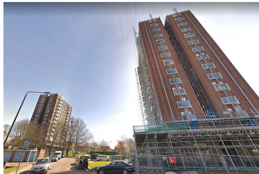
Many London local authorities have to invest in building safety improvements for their own stock (Picture above: the Granville Road tower blocks in Childs Hill during recladding, Source: Google)
