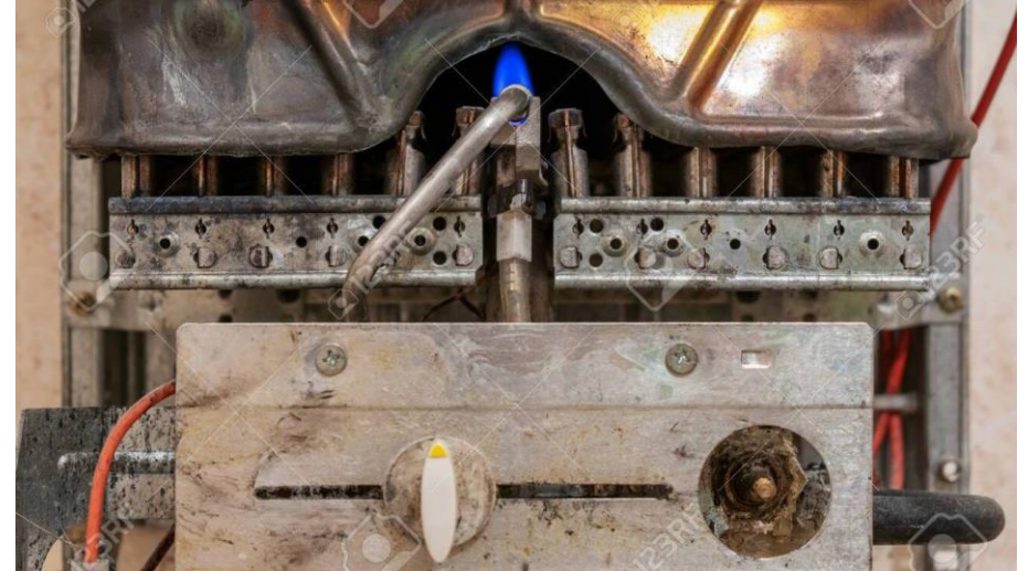
A number of gas boilers are coming to the end of their lives each year and their replacements are already covered by long term replacement and maintenance plans. We recommend a review of these plans and budgets in favour of low carbon heat.
